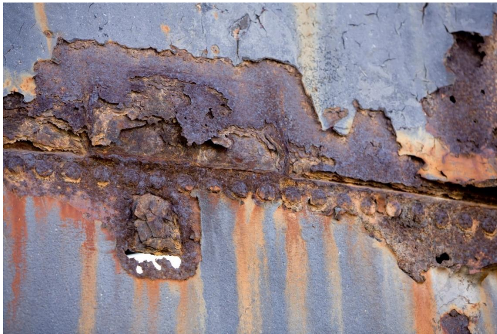
Figure 15 Crevice corrosion in practice. 43
