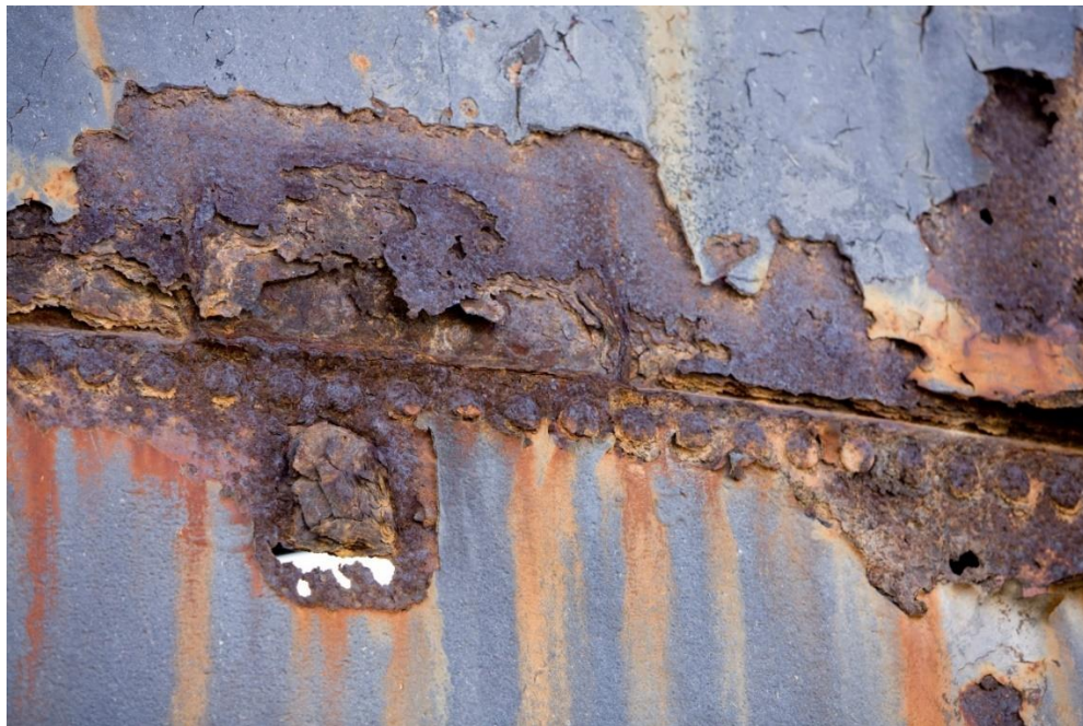
Figure 15 Crevice corrosion in practice. 43
