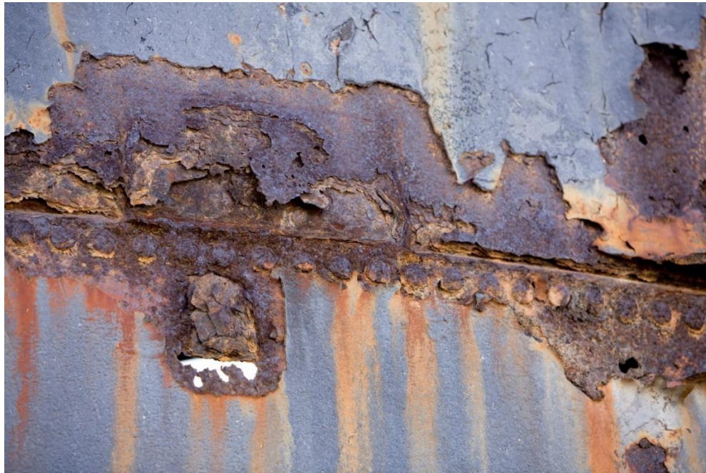
Figure 15 Crevice corrosion in practice. 43
