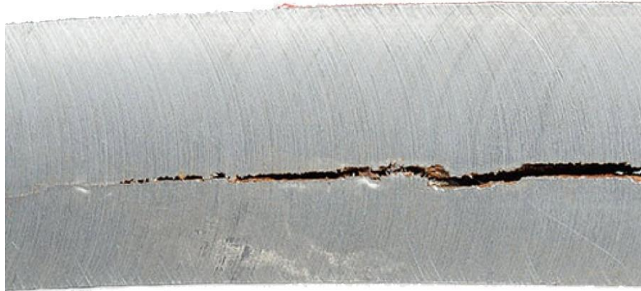
Figure 17 Stress corrosion cracking in stainless steel. 46
